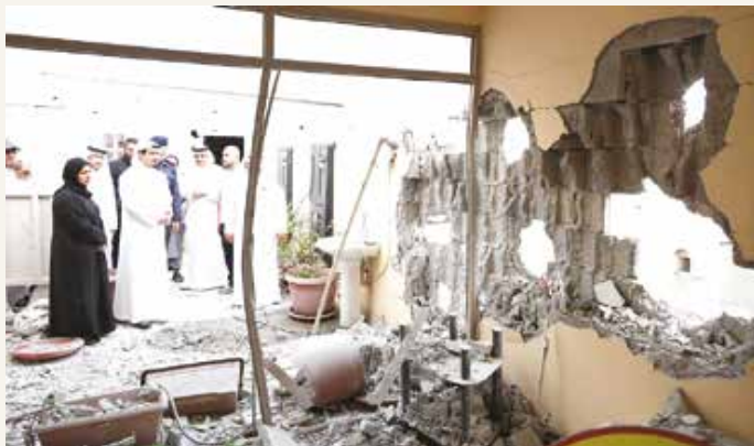
Plate 1 · Wall openings, exposed masonry and scattered debris are visible. Image extracted unchanged from The Daily Tribune, 10 March 2026, p. 4. [6]
